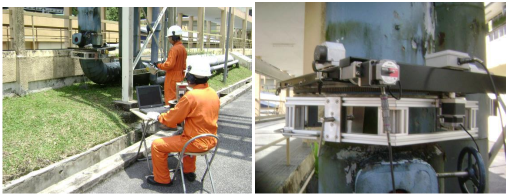
Figure 1: Portable clamp-on gamma-ray tomography system installed on a pipework
